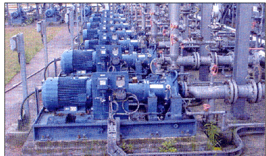
Pumps installed in a major overseas refinery
